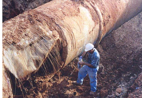
Figure 13. Failed section of 66 inch diameter pre-stressed concrete cylinder pipe.
