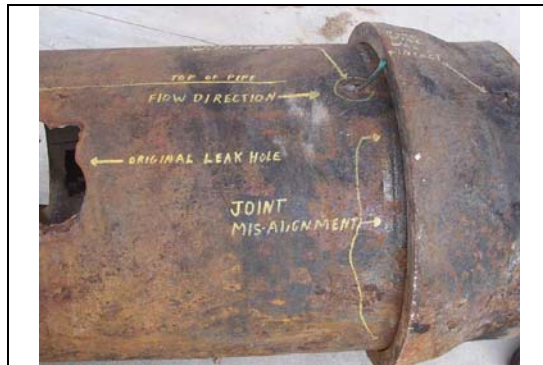
Figure 5. Failed region on pipe with detailed information written on pipe to show the original leak hole, misaligned joint, direction of flow and where the hole was on the pipe (e.g. top or bottom).
