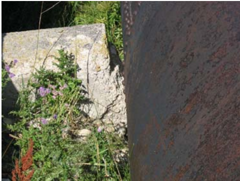
Figure 10. Cracked and deteriorating concrete saddles leading to sagging of the pipe, added stress on the joints, and damage to the coating on Halls Coulee Siphon. Also shows deteriorated coating on pipe.
