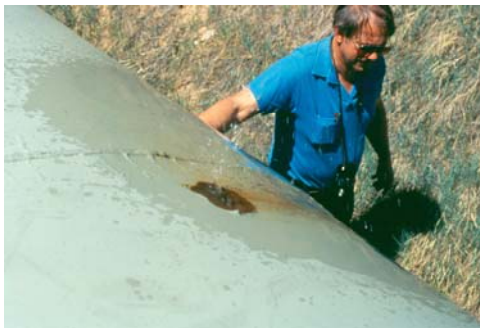
Figure 3. Leak on an elevated coated and lined pipeline.
