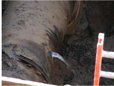
Figure 2. Perforation resulting from corrosion of a pipeline.
