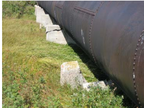
Figure 11. Cracked and leaning concrete saddles leading to added stress on the joints and damage to the coating on Halls Coulee Siphon.
