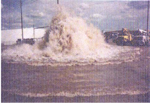
Figure 12. Failure of a 66 inch diameter pre-stressed concrete pipe.
