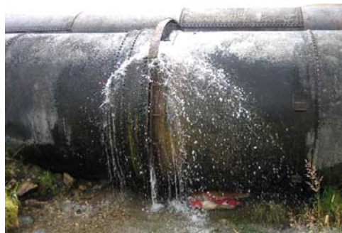
Figure 4. Leaking joint on elevated section of Halls Coulee Siphon.
