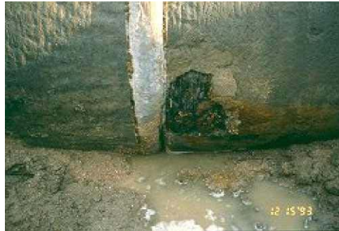
Figure 14. Spalling of the mortar coating on a pre-stressed concrete pipe which could eventually lead to failure of the pipeline.
