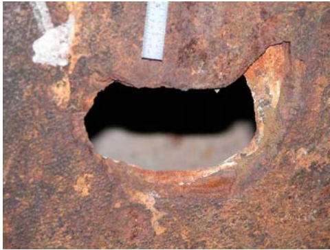
Figure 6. Hole in pipe with dimensional scale shown using a ruler.
